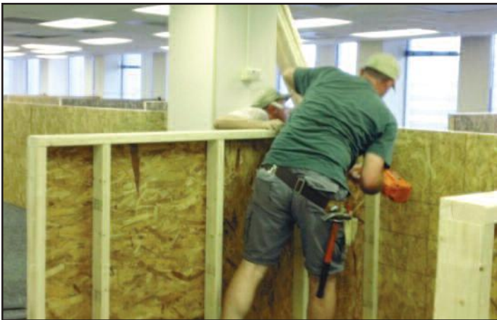
Figure 2: Office cubicle props on fire floor (10th)
