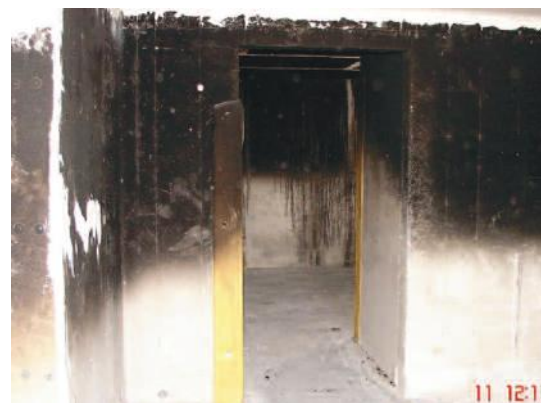
Figure C-7: Interior View of Burn Prop
